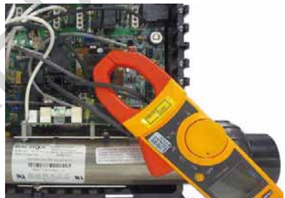
WHEN TESTING AMPERAGE
