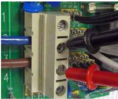
Brown to Blue Wires on a 230V BP2100 System
