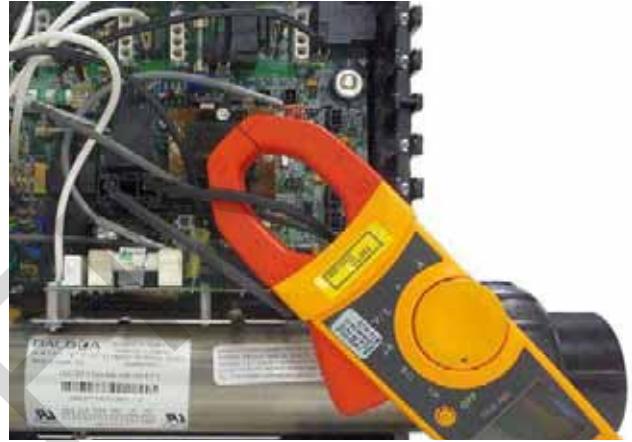
AMPERAGE HEATER TEST BP2100G1
